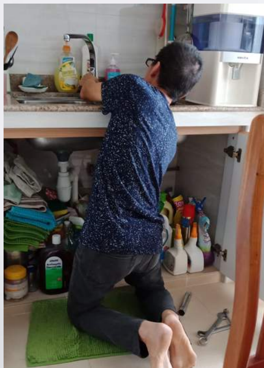
A HMS volunteer carrying out basic plumbing works in a senior's home.
